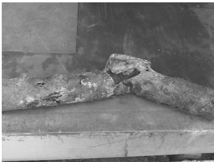
Fig. 1. Damage of gas pipe caused by an external company during trenchless drilling [5]
