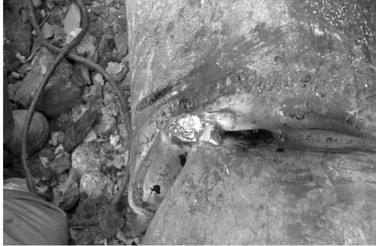
Fig. 2. Damage of gas pipe caused by the mining impact [5]
